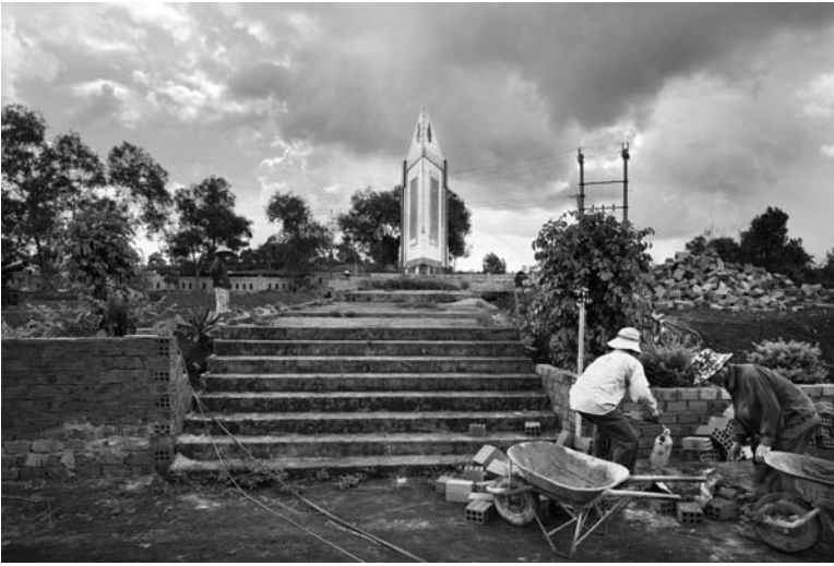
Fig. 5. War memorial under construction at Khe Sanh, site of one of the most legendary battles of the American War in Vietnam. Building new memorials and museums, and renovating old ones, is an ongoing process in the country. Courtesy of Sam Sweezy.
